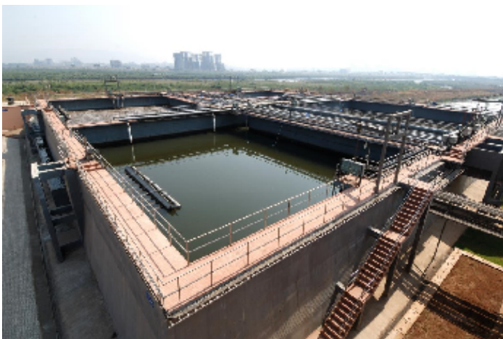
Figure 1: KAHRGHAR STP 4 BASIN MODULE, 25 MLD design
